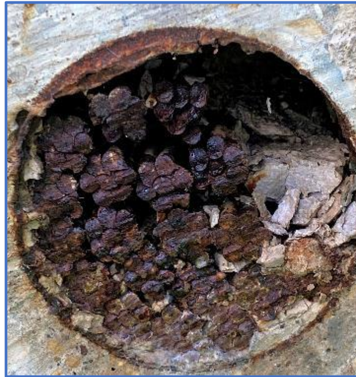
Corroded strands in a poorly grouted duct
