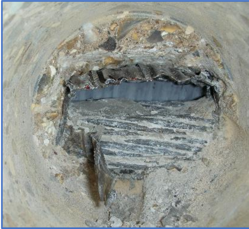
Lack of grout in post-tensioning duct
