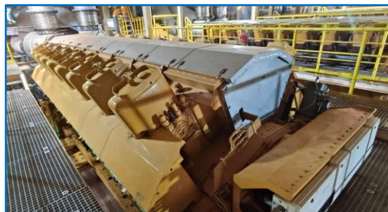
10 engines in Tokadeh powerhouse
