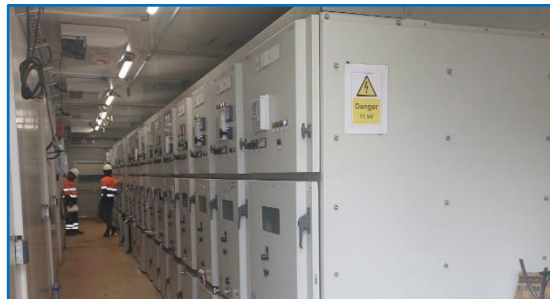
Next-generation control room & E-house
