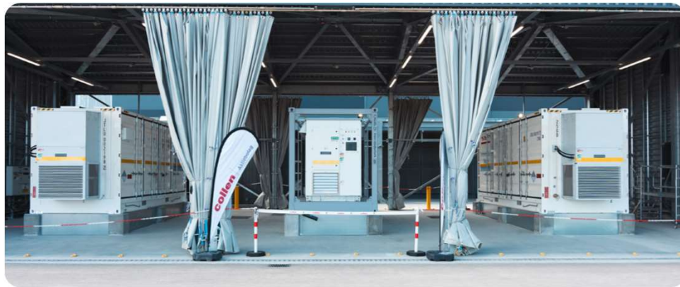
2 battery containers + PCS/MVPS + microgrid controller
