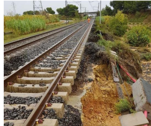
Landslide due to bad weather
